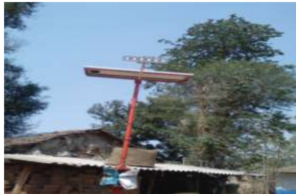
Solar Streetlight at Chondipada
