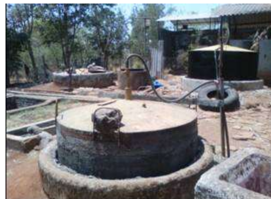
Floating dome biogas plant operating with de-oiled cake as feed material
