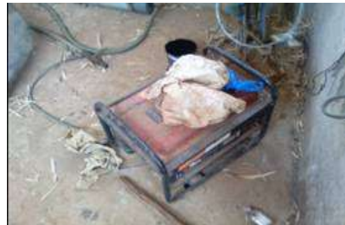
Biogas operated portable genset at Jawhar school
