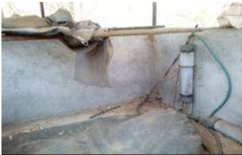
Rubber Balloon for biogas storage at Jawhar school
